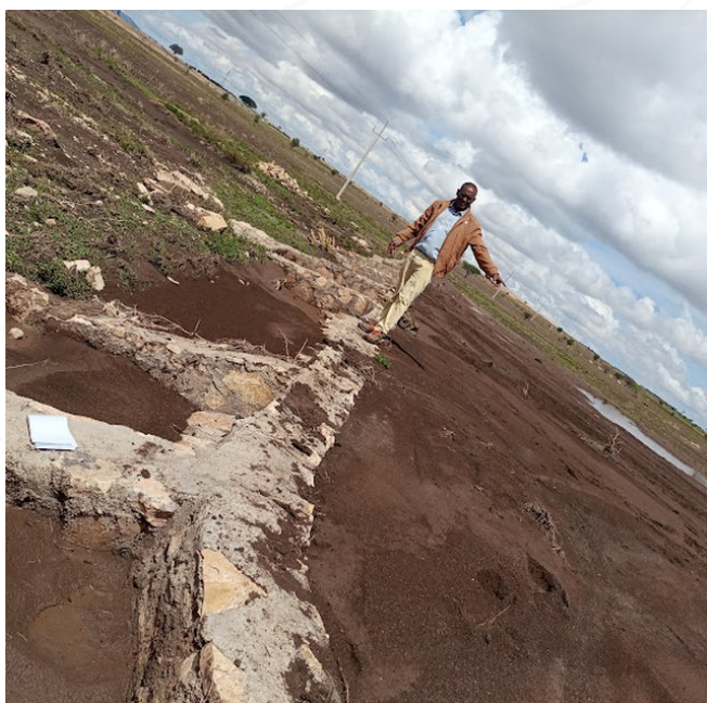
The sediment and water arrested by WSW right after the first shower. The rainwater is harvested and spread in the farm along the length of the structure. (Gerba Leta)
