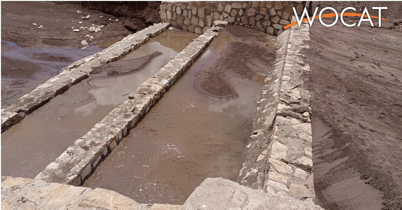
Double basin Masonry Check Dam where massive amounts of sediment are trapped by the structure (Gerba Leta)
