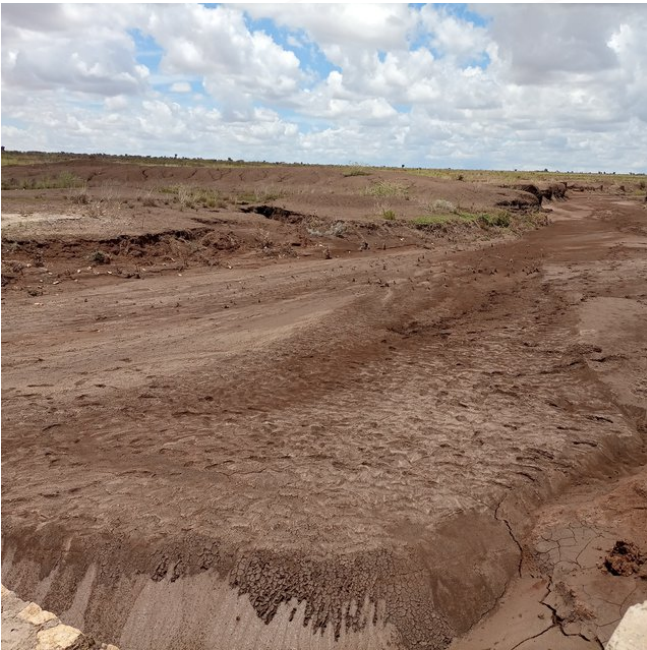
Massive sediments and debris trapped behind the recently built structure. (Gerba Leta)
